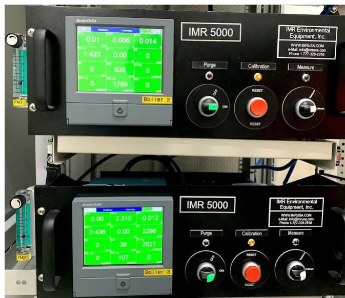
CEMS IMR 5000 19" Racks
